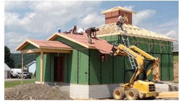
Shingles are installed upon the roof of the new chapel on July 20. To see a full gallery of construction photos, visit holyspirit-oca.org .
